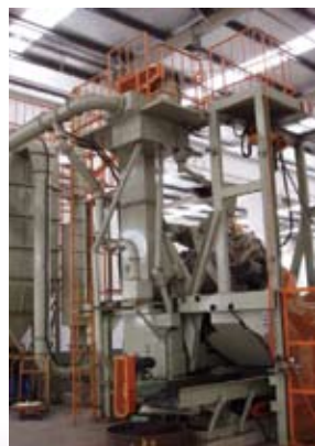
鍛造設備 Forging equipments
